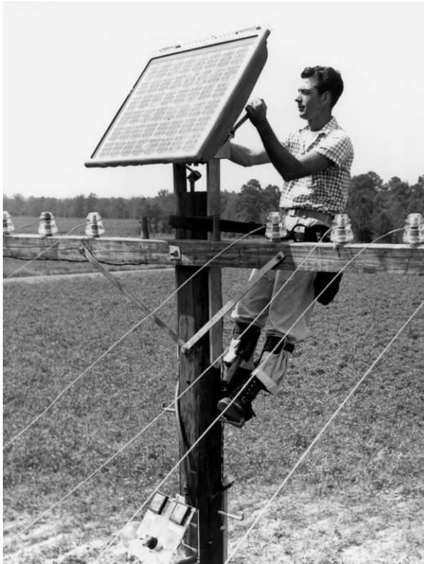
Adjusting the Bell Solar Battery to make the first sun-powered telephone call in 1955
